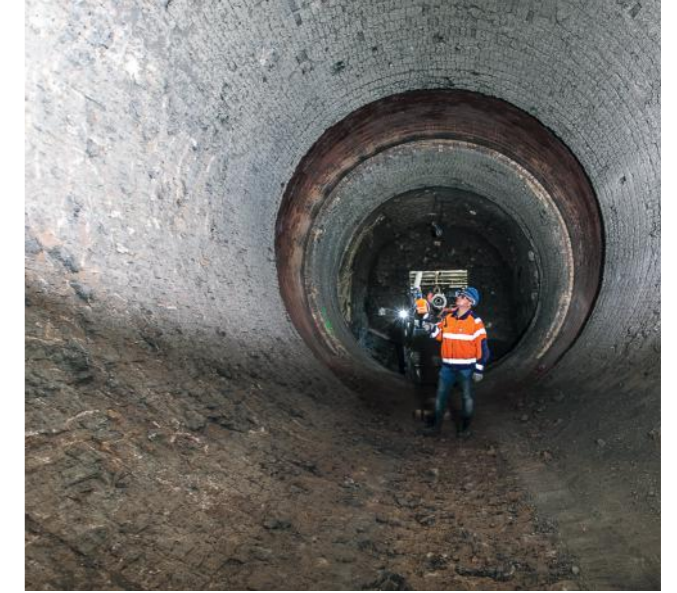
→ Photo of VICAT/Peille - Kiln interior
