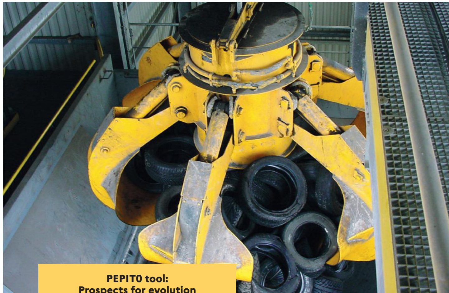
→ Photo of VICAT/Alternative Fuels - Storage of whole tyres - Lifting grapple
